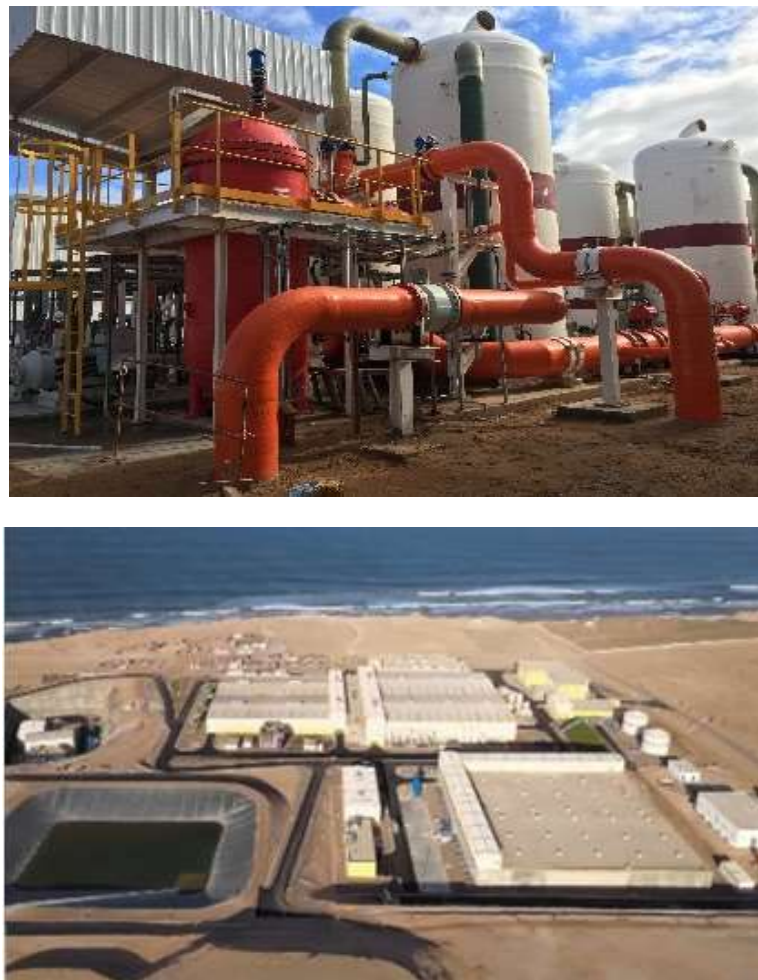
Figure 6. Morocco desalination plant reverse osmosis industrial infrastructure Right: Overview Left: Equipments
